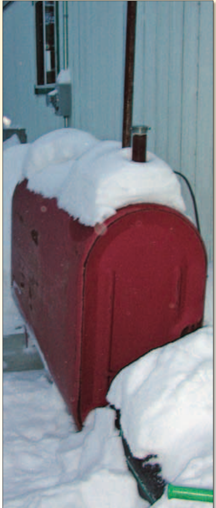
Typical oil tank location.
