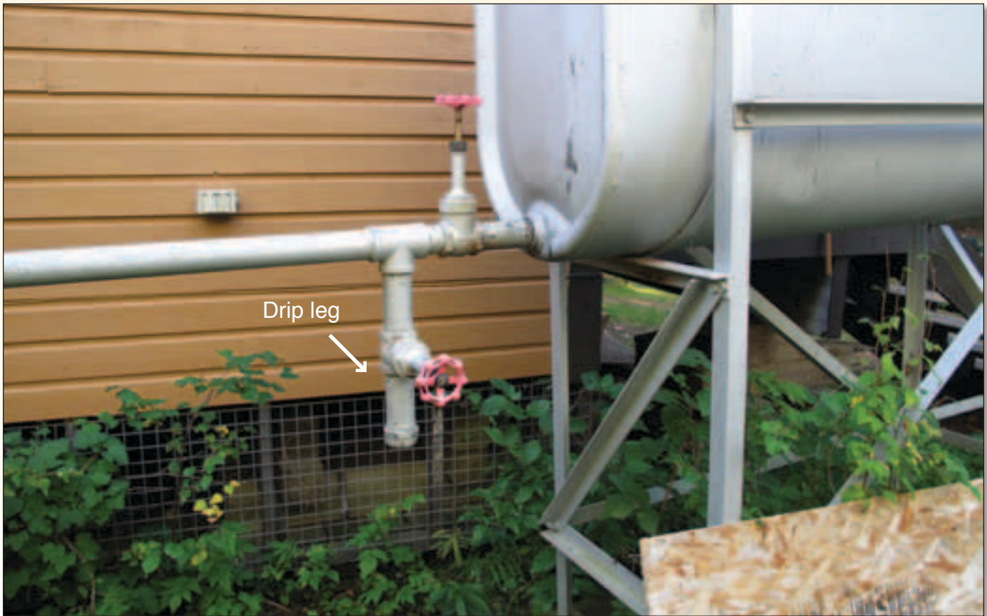
Drip leg extends below the level of the fuel line.
