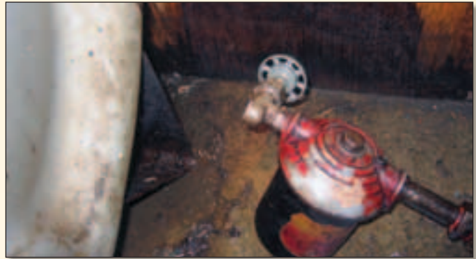
Broken valve on oil tank in basement.
