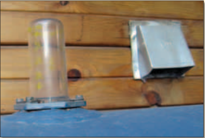
Oil level gauge. Note the empty tank.
