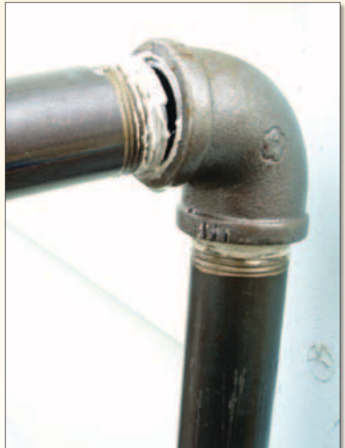
Broken fuel line at elbow due to stress from shifting oil tank.
