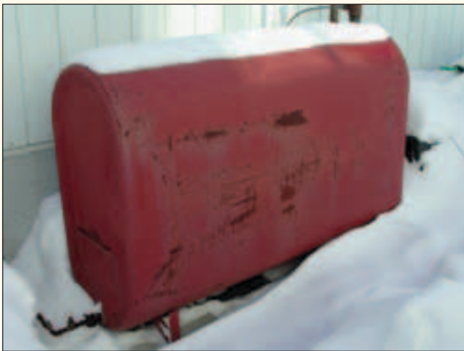
Single-wall, 1,135 litre (250 gallon), heating oil tank. Note the surface rusting.
