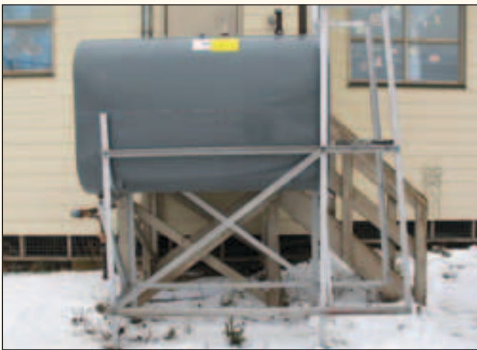
Epoxy-coated, 1,135 litre (250 gallon), single-wall steel heating oil tank on metal tank stand.
